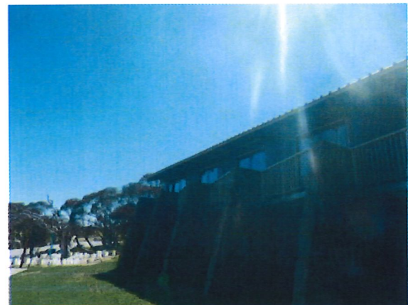
Figure 6: Photo of the northern elevation and bedroom wing - location of replacement cladding on the ground floor (below windows) and boxing of the eaves
