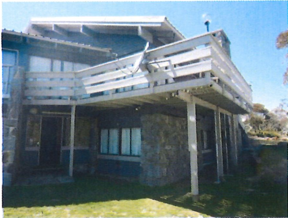
Figure 3: Photo of the timber deck to be replaced and enlarged with a steel deck, with external steel fire stairs
