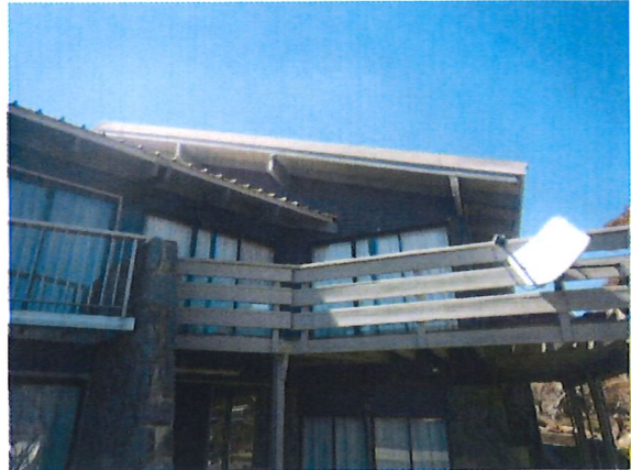
Figure 4: Photo of the floor to ceiling windows to be replaced with smaller windows
