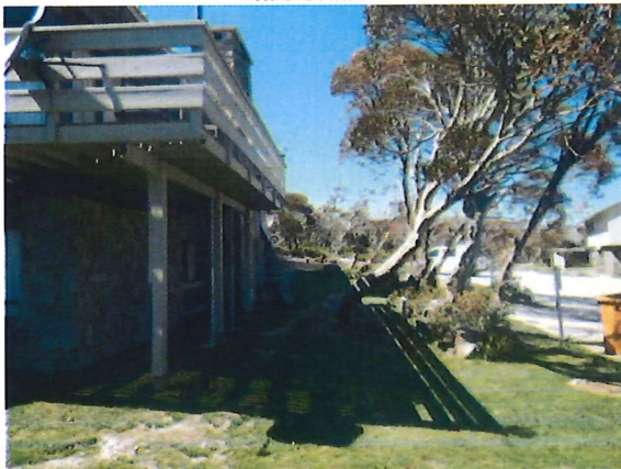
Figure 5: Photo of the deck to be replaced and enlarged, with external fire stairs
